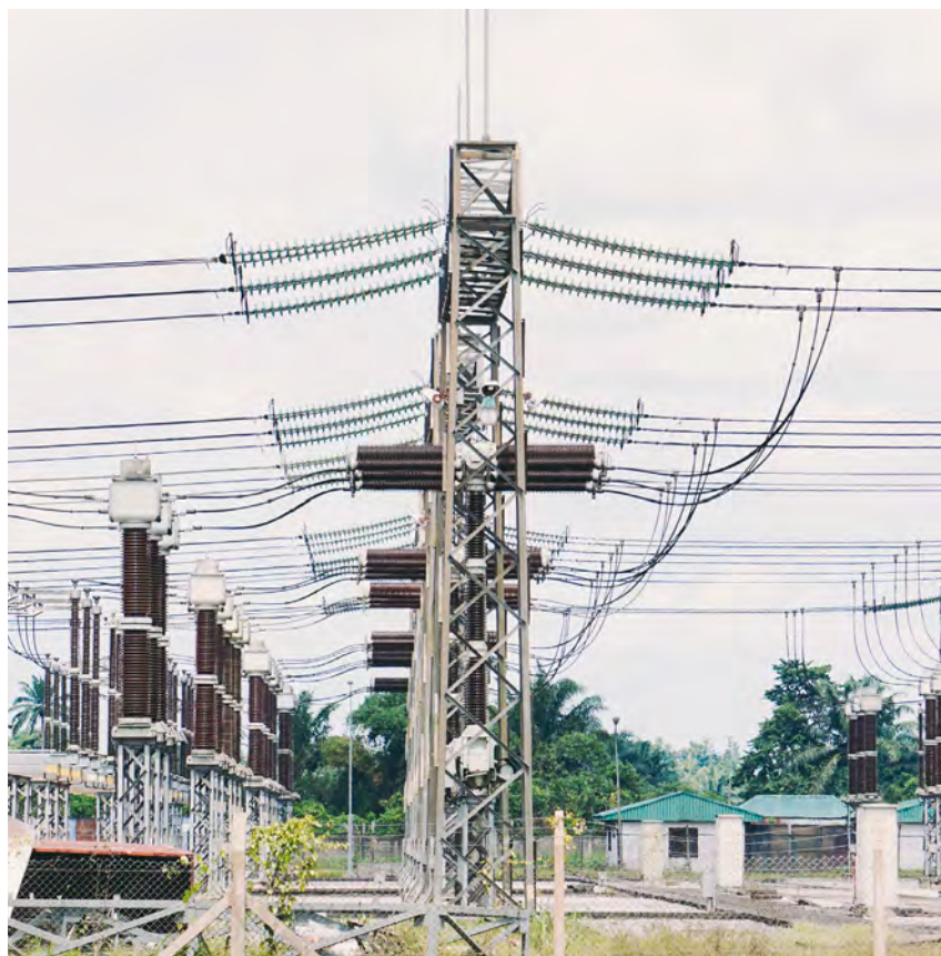
A side view of the transmission lines from Transcorp Power plant.
